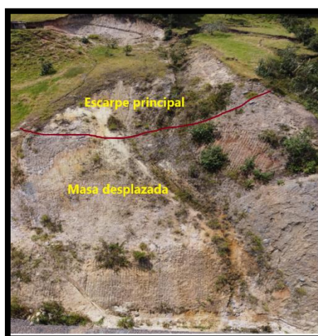
Figura 76. Deslizamiento 2. x: 744503,60; y: 9657899,56; z: 2819,8
