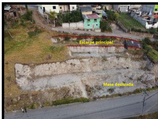
Figura 86. Deslizamiento 12. x: 745269,914; y: 9662790,650; z: 2503,77
