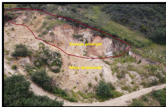
Figura 79. Deslizamiento 5. x: 744614,217; y: 9658801,687; z:2638,55
