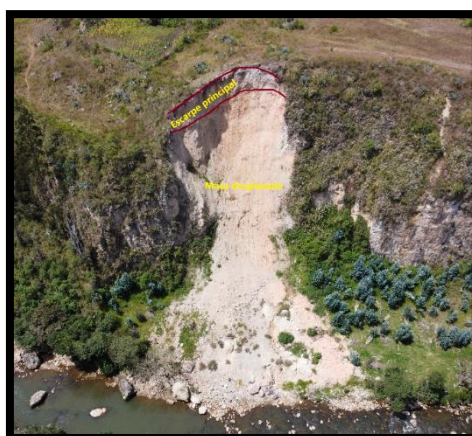
Figura 89. Deslizamiento 15. x: 744117,470; y: 9665938,794; z: 232822
