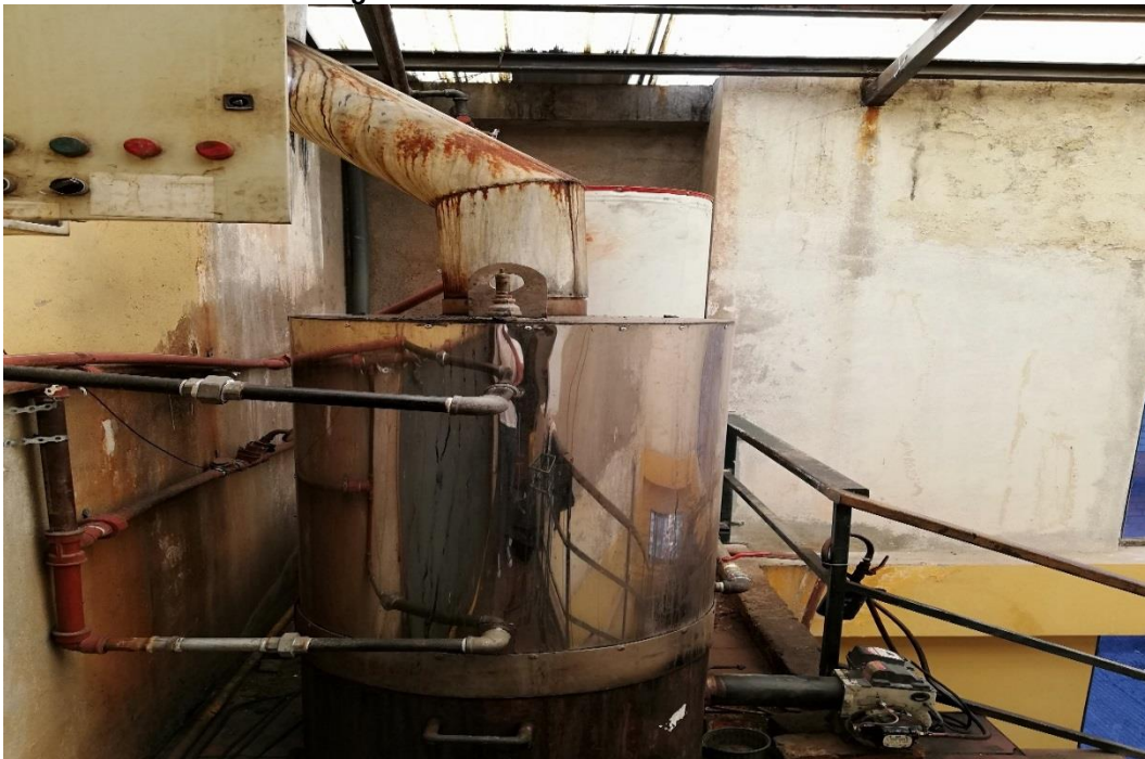
Figura 46 Caldero Industrial Hotel Bombuscaro
