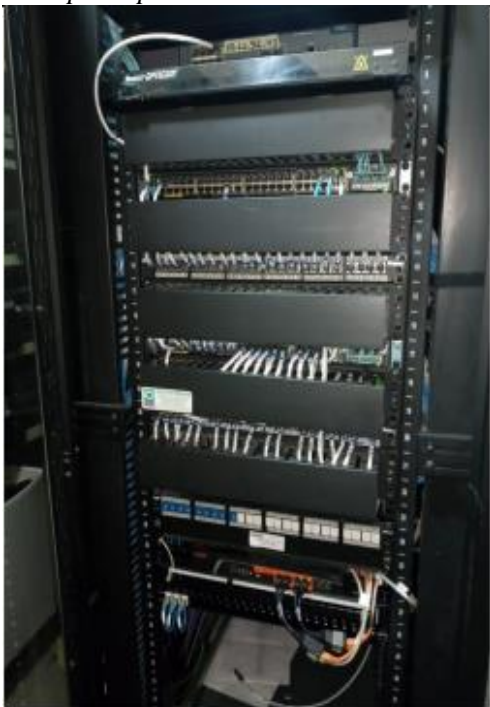
Figura 15 Rack principal del HGMYM
