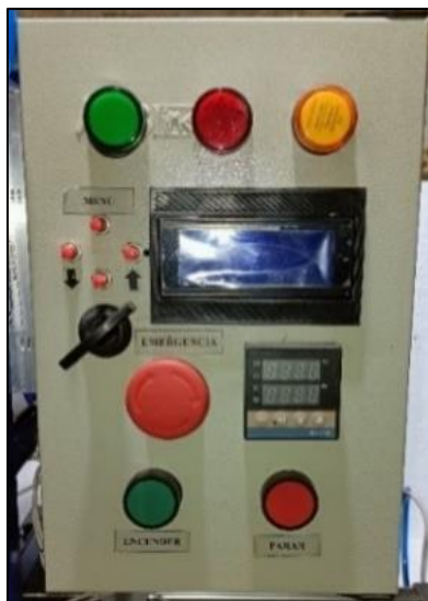
Figura 93. Panel de control.
