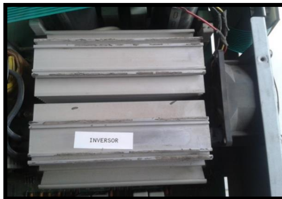
Figura 23: Inversor incorporado al ups
