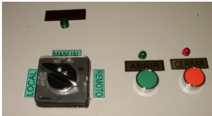
Fig. 3.13 Panel de control
